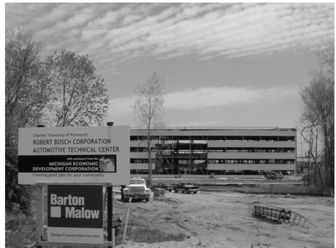
Construction of the Robert Bosch Corporation Automotive Technical Center began in 2006. Located on Five Mile Road and Haggerty Road, it is expected to be operational in 2007.
