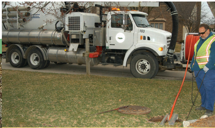
FOG build-up in sewer pipes (shown below) is costly to clean requiring local public works staff to go to the site and remove the blockage (shown above).
